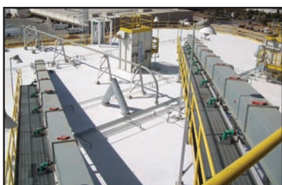
Aeration conveyors feeding multiple silos.
