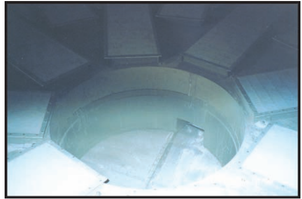
Aerated bin bottom silo discharge.
