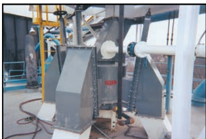
Aerated distribution box with four discharges.
