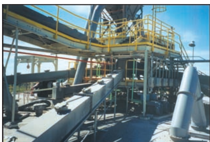
Aeration conveyor run.
