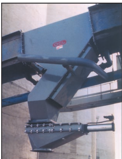
Aerated lump trap with slide gate valve.
